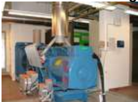
Emergency powersupply for a hospital in Austria
