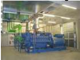
Emergency powersupply for a hospital in Austria
