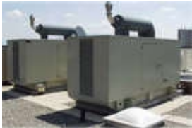
Emergency powersupply for a Pharmaceutic Company
